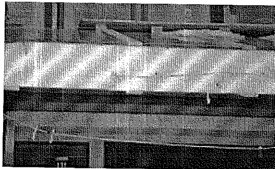
This is a photograph of the cracked exterior deck roof beam at unit ?.
